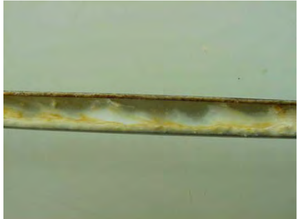
Scale Build-up in Tubing
